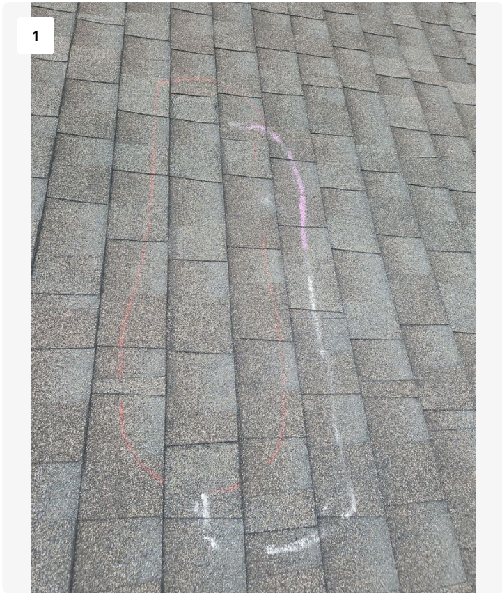
Each shingle circled is delaminated and lifts allowing debris and moisture underneath
